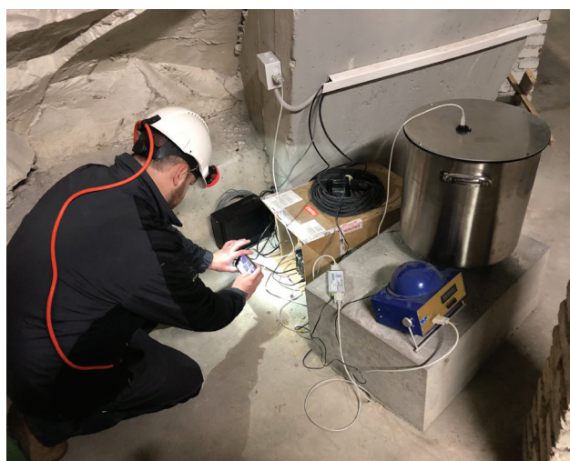
Installation of Rotaphone station near Litoměřice
